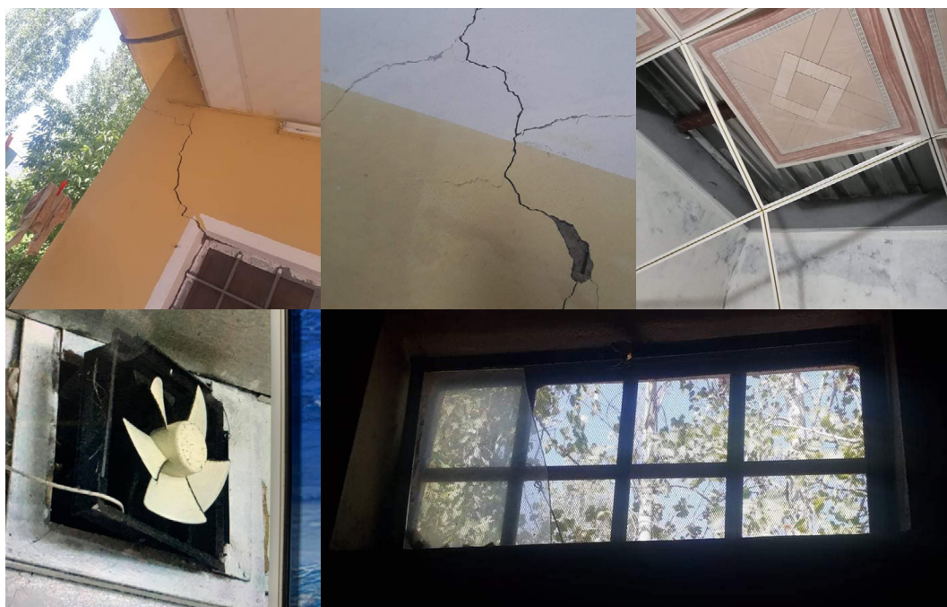
Damage to property following shelling between Sept. 17-18 in the village of Chalik, including cracks to exterior and interior walls, a displaced wall fan and ceiling tiles, and broken windows.
