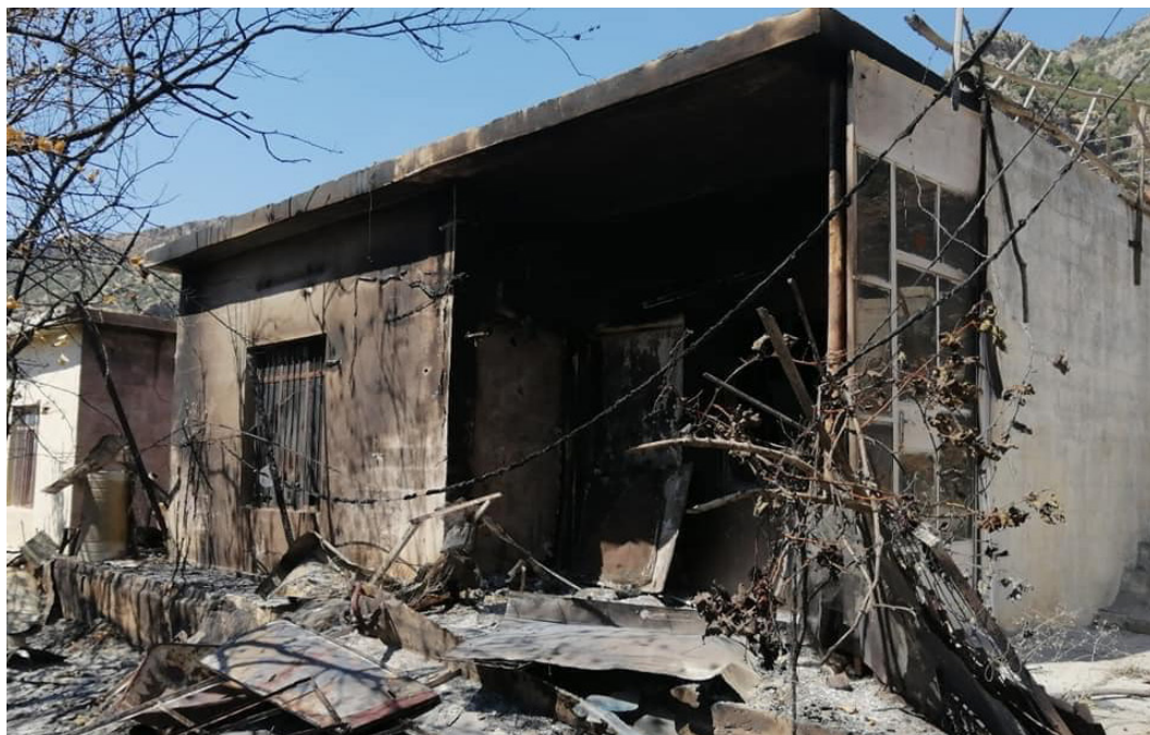
A damaged home in Sharanish following shelling near the village. (Sept. 10, 2020)
