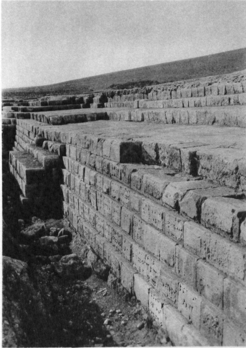
A.—The repaired breach, showing re-used stones inscribed with parts of inscription D
