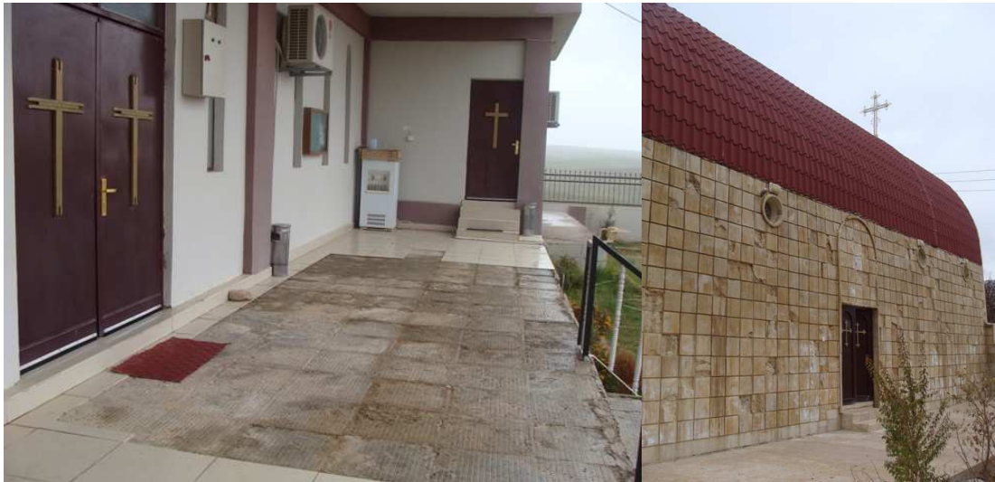
Churches by Aghajan and the KRG: St. George’s Ancient Church of the East in Bakhitme (left). Not only has the paint peeled off the dome, but the floor tiles have also come loose. At St. Sawa’s Assyrian Church of the East in ‘Ayn-Nune (right), the marble facade has dangerously cracked and is collapsing.
