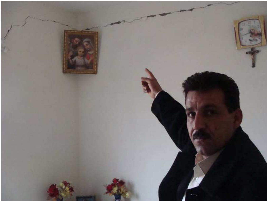
Homes by Aghajan. A worried Assyrian man in Shiyoz points to the cracks in the walls of his foundation-less, and shoddily built house.
