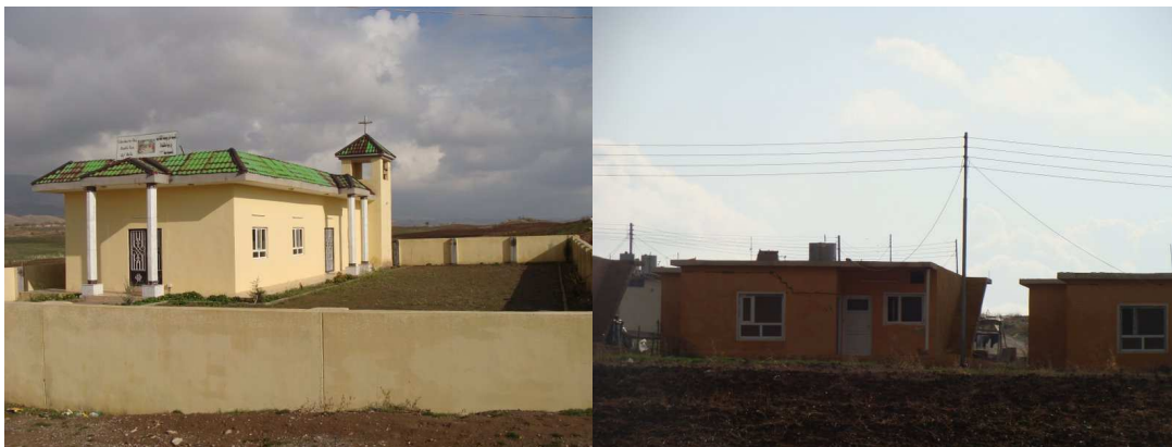
At oil-rich but impoverished Navkandala, not only have the roof tiles of the Aghajan-built church gone green (left), but many of the houses (right) are so dangerously cracked they are practically uninhabitable.
